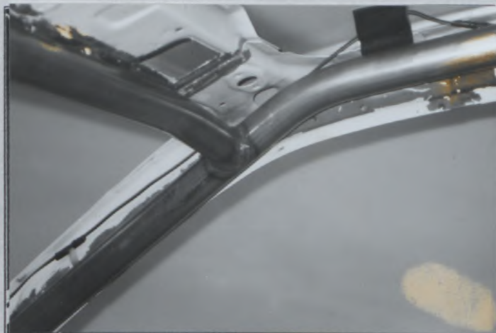
PHOTO No. 2 Lateral bar to A-pillar
