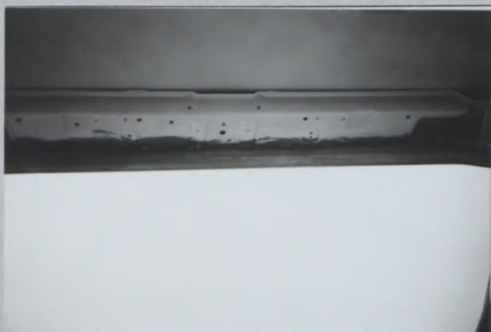
PHOTO No. 3 Front screen bar to roof
