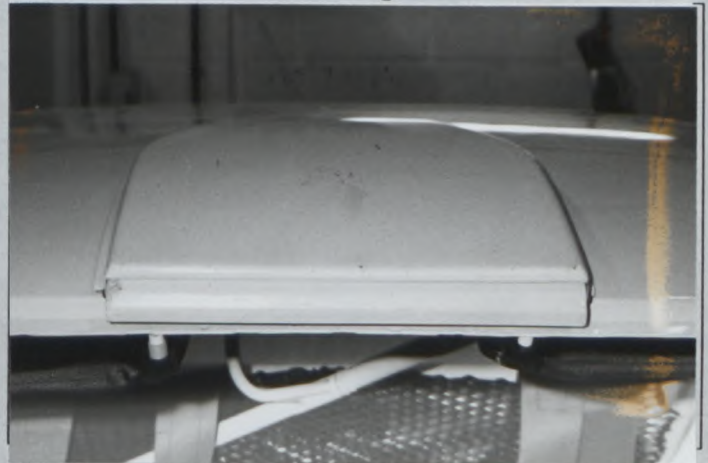
PHOTO No. 98 FLAPS FOR VENTILATION
