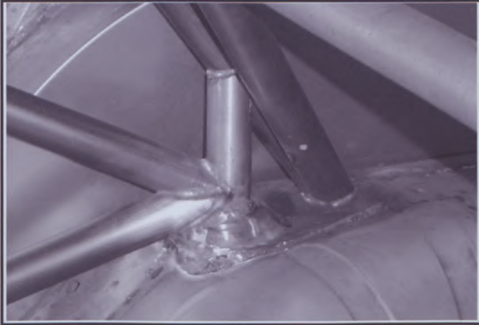
PHOTO N° 6 : Rear strut to floor
