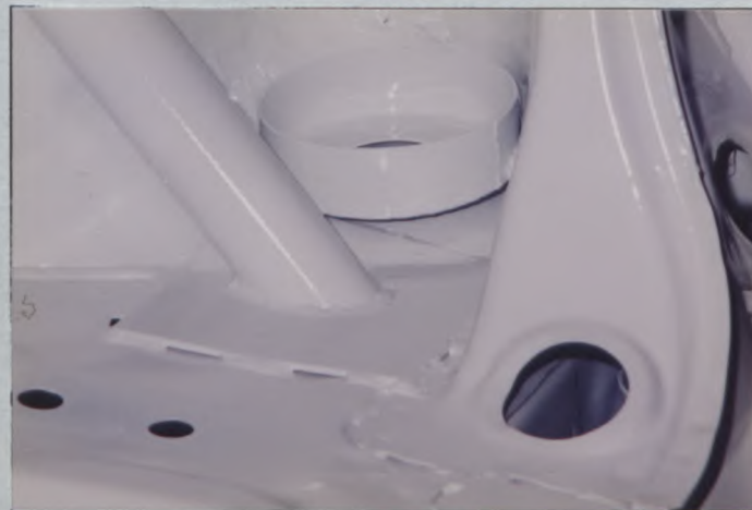
PHOTO No. 10 REAR SUPPORT BAR TO FLOOR
